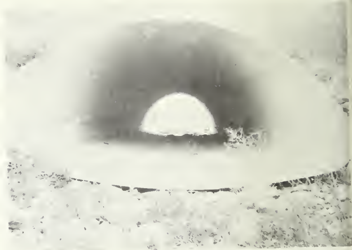
SOUTH ENTRANCE: Notice outlet erosion, boulders washed in other end
